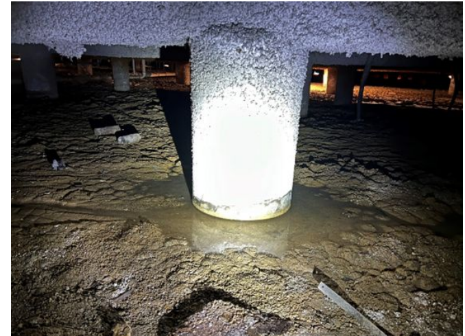
Crawl Space Water Infiltration
